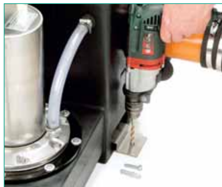
Assembly anti-buoyancy safeguard
